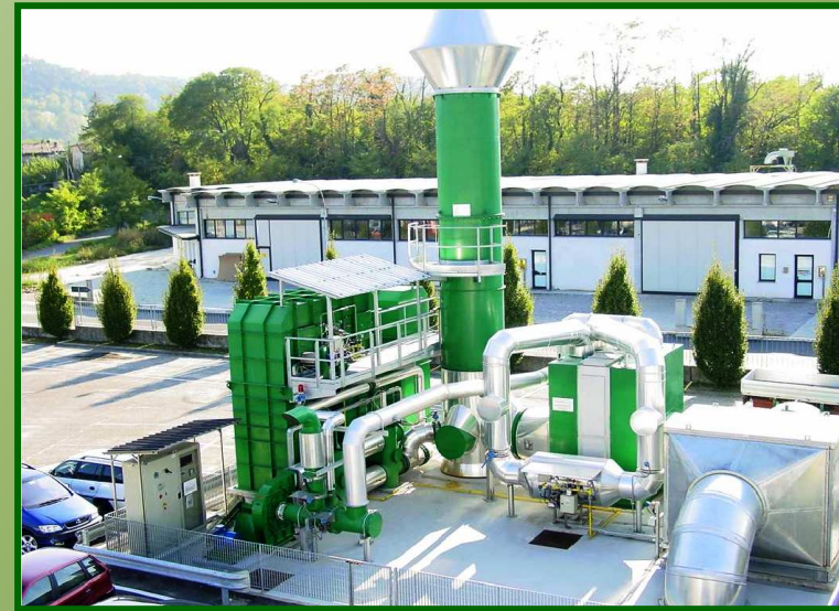
Rotor concentrator and thermal oxidiser RC & RTO
