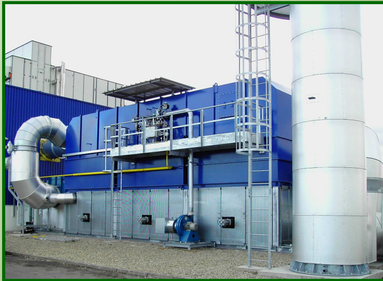
Regenerative thermal oxidiser – RTO
